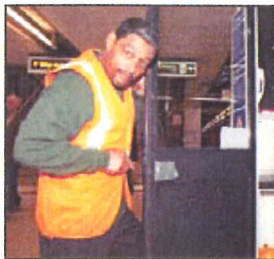
Running repairs: Roving handyman Carlton Chambers from contractor Acorn Projects fixes a loose door lock at Baker Street station
